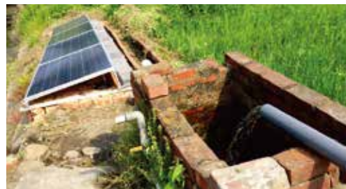
PV Water Pumping System
